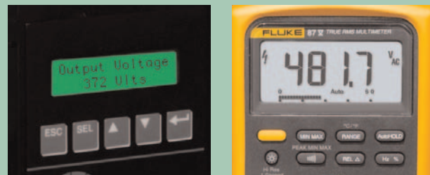
Figure 1. Output voltage reading without using the low pass filter.
